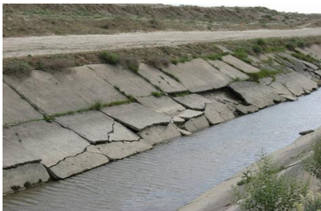
Figure 1. deteriorated rigid (concrete) veneer liner
