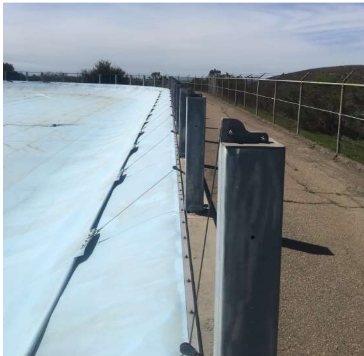
Figure 8. Mechanical Tensioning Tower System on Upper Valley
