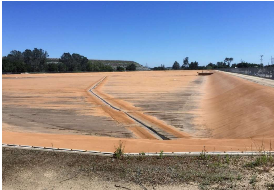
Figure 5. Hinkle Reservoir, 37-Year-Old CSPE Floating Cover Picture 2017
