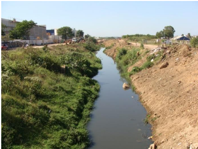
Figure 2. Current situation of the Passo da Mangueira initial stretch of the on Rua Dona Alzira, Porto Alegre.
