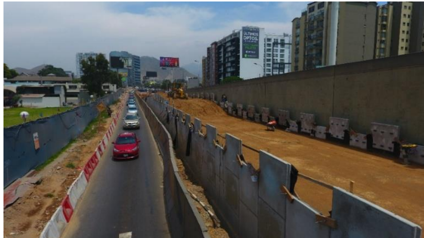
Picture N°6. Construction of the Reinforced Soil Wall – RI (Road Interchange) “El Derby”
