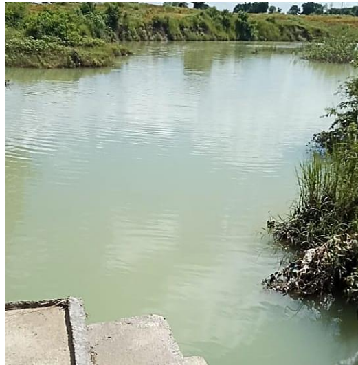
b) Reservoir behind the check dam after the second monsoon - 2019 (1.5 years post construction)
