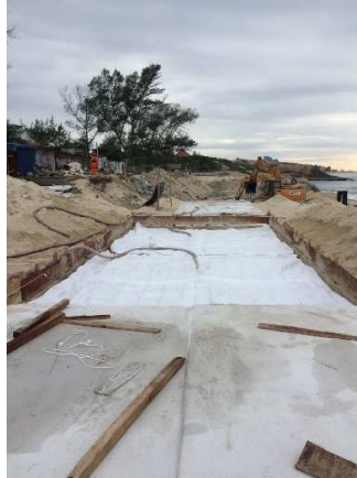
Figure 6 - Type 1 Section - Macumba Beach – Rio de Janeiro / RJ
