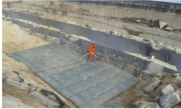
Figure 8 - Mattress filling with the concept of articulated concrete mattress – Macumba Beach – Rio de Janeiro
