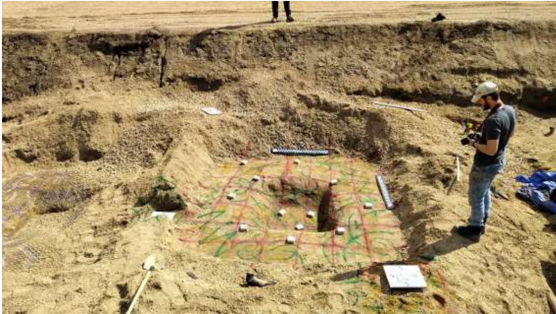
Figure 8: Forensic investigation uncovering underlying clay surface and geogrid
