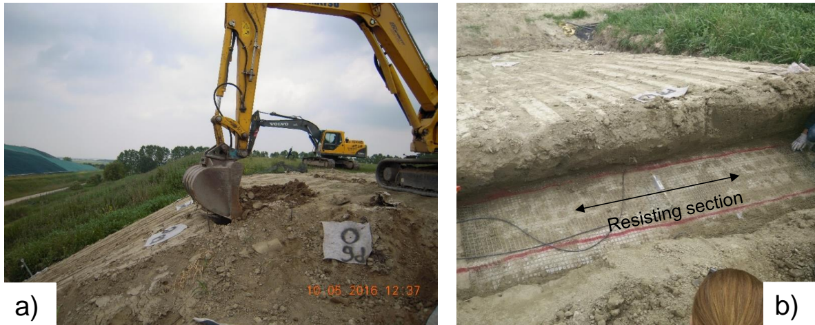
Figure 5. Induced failure phase: a) removal of the soil on top of the slope and; b) impression of the resisting cross-section after the cut of the geogrid.
