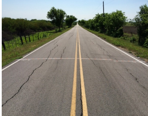
Figure 1. Typical longitudinal cracks related to expansive clays in pavements
