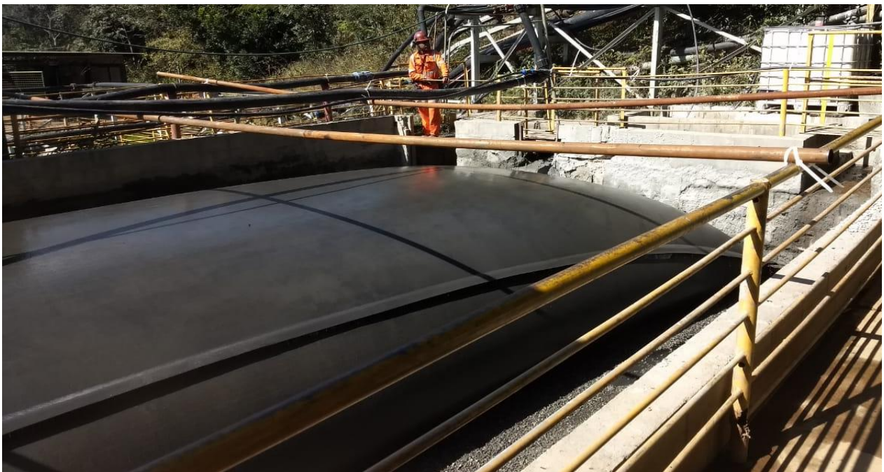
Figure 5. Waste confinement systems implanted in the place where the bays used to work.
