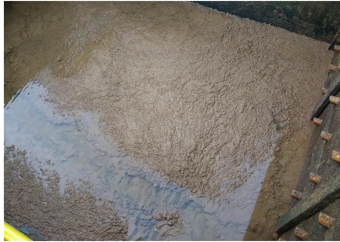
Figure 6. Decanter tank to be washed.
