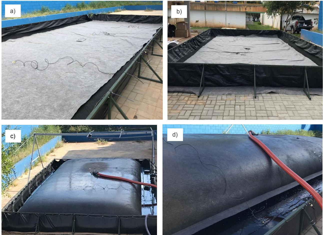
Figure 8. a. b. Waste confinement system ready for filling and accommodated within a metal structure with a geomembrane. c. d. Waste confinement system during a filling process.
