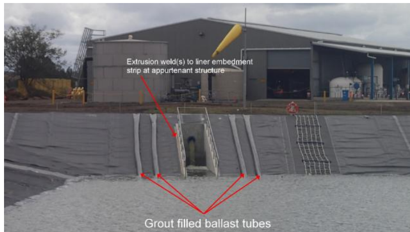
Figure 3. Grout filled ballast tubes assisting with minimising stress on extrusion welds to LES
