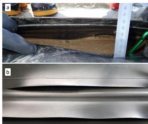
Figure 1. Photograph of Hole 1: a) top side; b) bottom side
