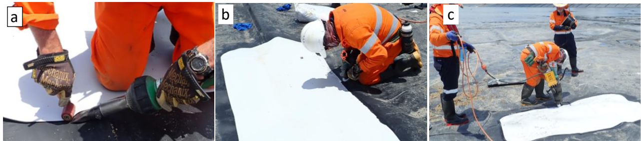
Figure 6. Photographs showing the sequence of patching: a) temporarily heat bonding; b) grinding; c) extrusion welding
