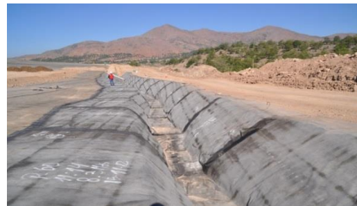
Figure 9. Leachate collection canal
