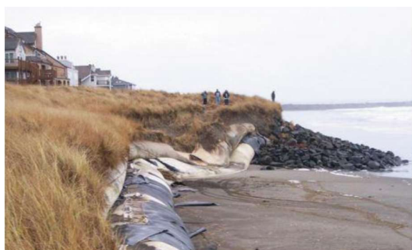
(g) damage – overview 5
