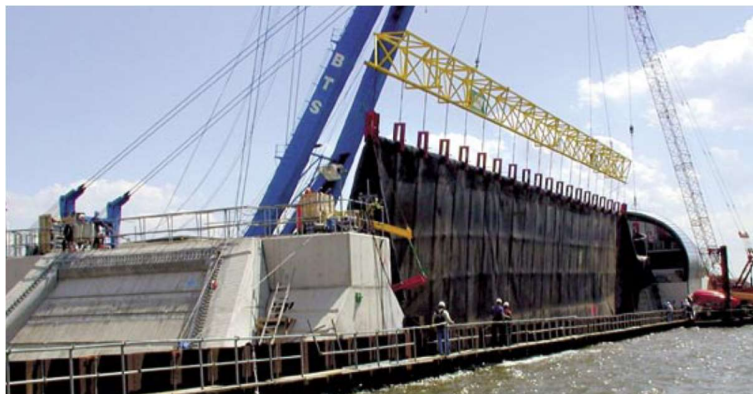
(a) storm barrier consisting of geomembrane
