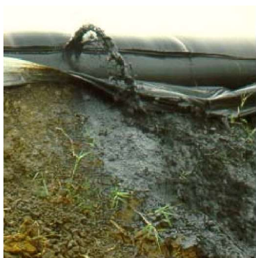
(a) local rupture – overview 1
