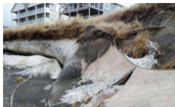
(h) damage – detail 5
