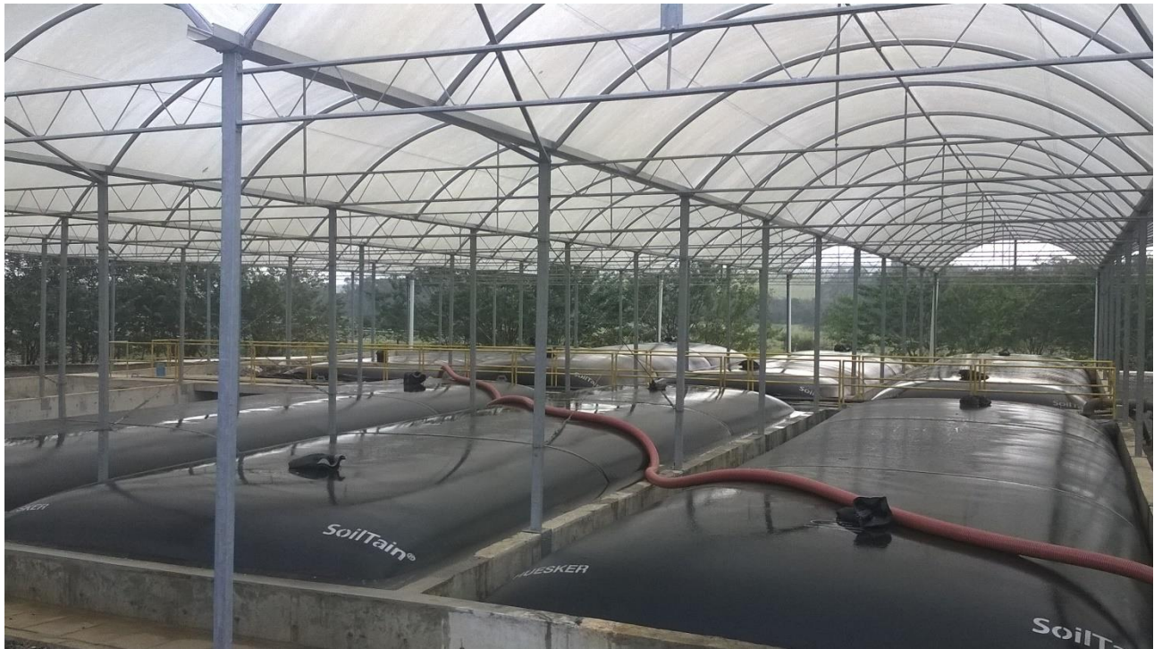
Figure 3. Geotextile tubes located in the drying beds (Authors, 2019).
