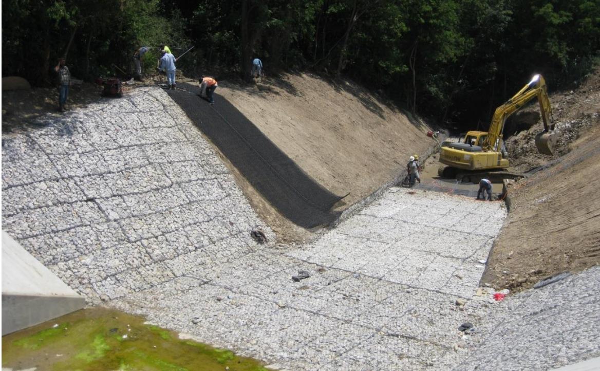
Figure 7. Installation of DTWM reinforced geomat on steep creek banks and connected to gabions.
