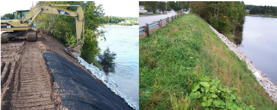
Figure 2. Geomat with DTWM reinforcement on a steep soil slope before and after the establishment of vegetation
