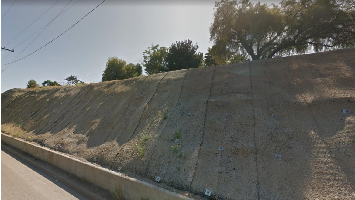
Figure 5. Soil Nailing system with DTWM reinforced geomat and hydromulch before growth of vegetation.
