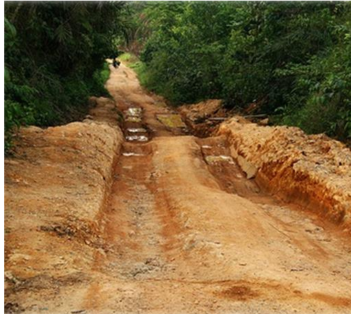
Figure 3. Effect of traffic and loads on an unpaved road on weak soil.
