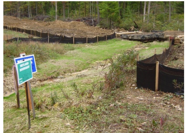
b) Geosynthetic silt fencing
